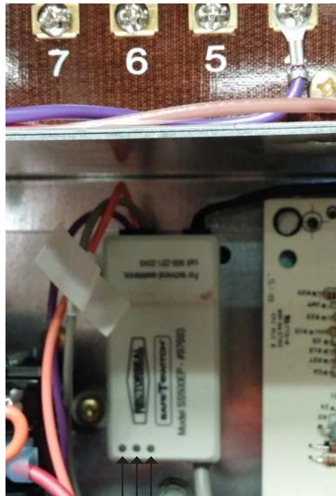
FIGURE 36 Outdoor Condensate Control
