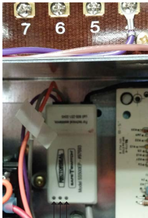
FIGURE 19 Outdoor Condensate Control
