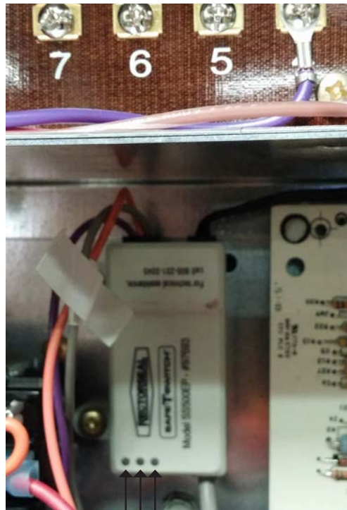
FIGURE 19 Outdoor Condensate Control
