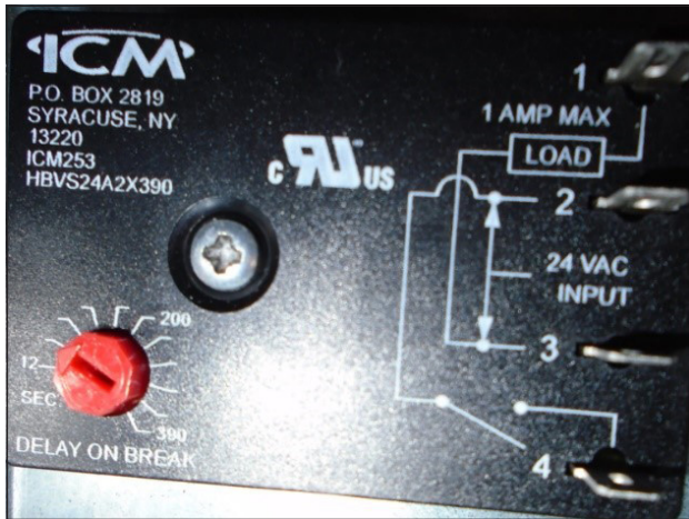
FIGURE 4 Exhaust Fan Off Delay Timer
